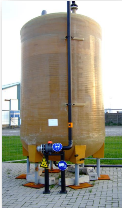
Addition of chemicals
