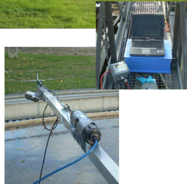
TSS and velocity sensors used for profile measurements
